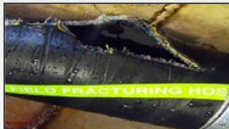
Hose assembly rated to 400 psi.
